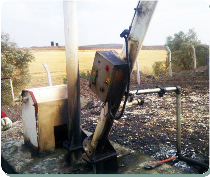
Damaged Flare Stack
